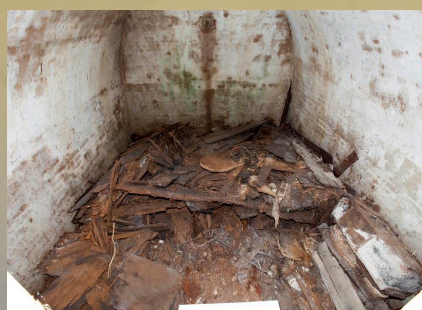
Figure 2. Collapsed shelving and deteriorated coffins inside the Causten family vault.
